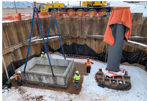
Dry well access tube and placement of pig launch vault base in the excavation
