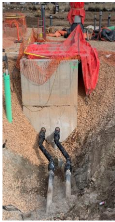
Two 8" force mains connected to pig launch vault
