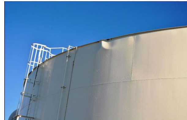
Existing Reservoir Deformations
