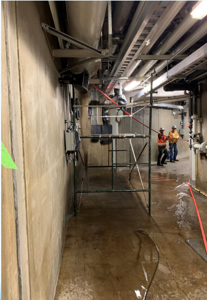
CVWRF Tunnel System – Staff aiding with sludge line cleaning within the structure.
