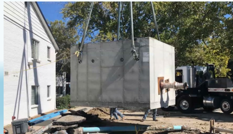
Large Meter Vault
