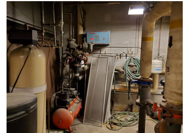
Illegal connections – hoses attached to fire riser piping
