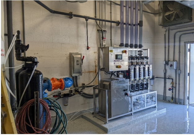
Well No. 15 Chlorinator installation
